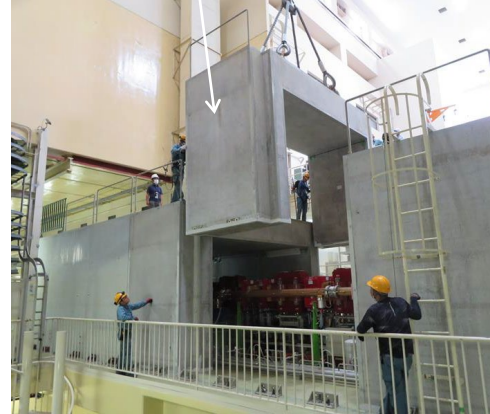
Concrete radiation shield
