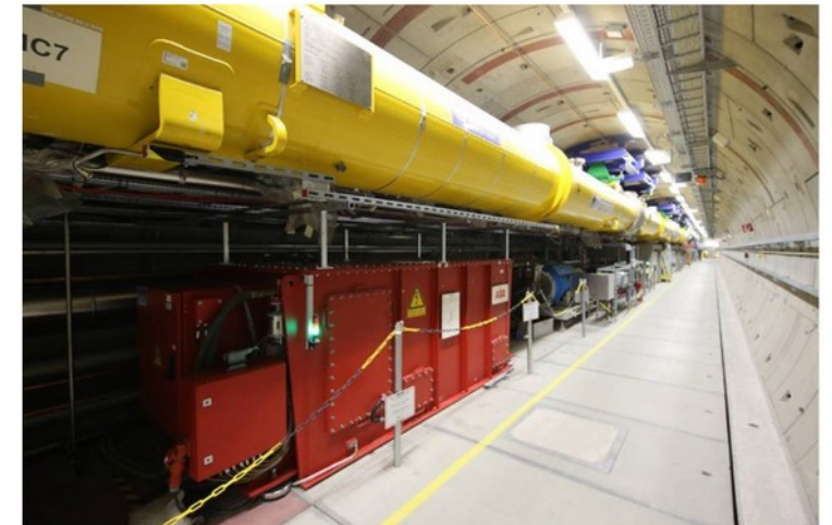
Figure 3: RF station in the E-XFEL tunnel.
